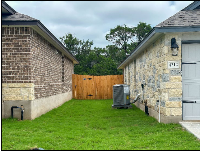
Left: Wooden fence attached directly to structure
